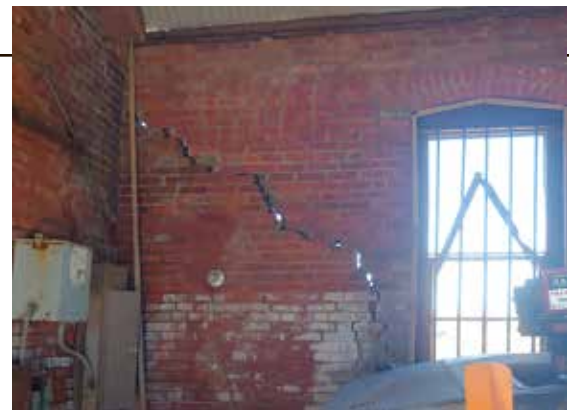
Masonry repairs needed at Fort Delaware State Park
