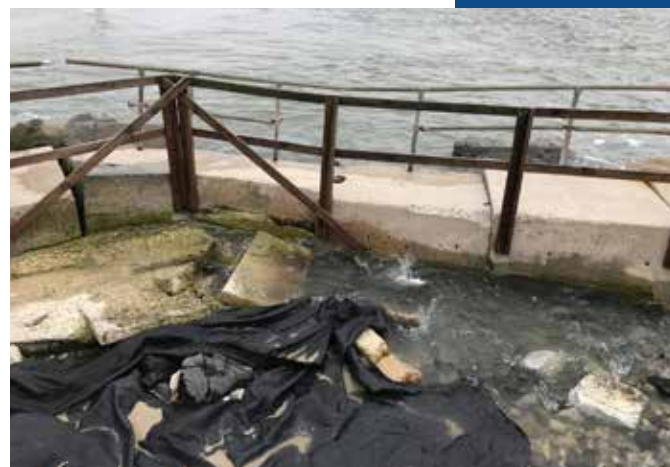
Erosion of the jetty under the Indian River Bridge at Delaware Seashore State Park
