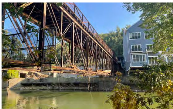
Bancroft Bridge damage at Alapocas Run State Park
