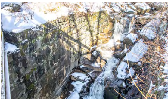
Stone wall damage at Alapocas Run State Park
