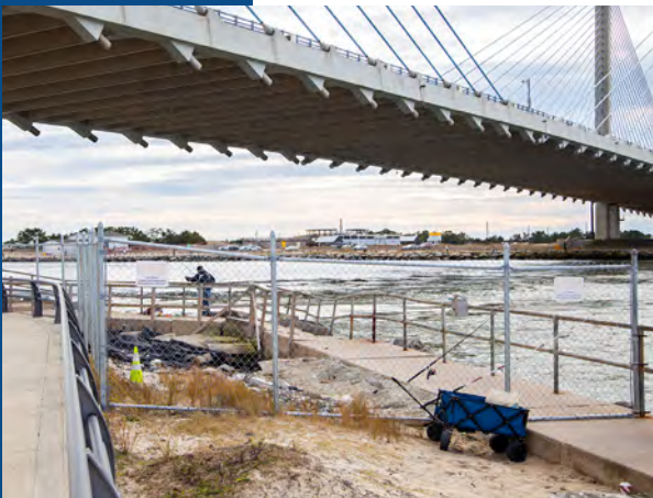
Erosion of the jetty under the Indian River Bridge at Delaware Seashore State Park
